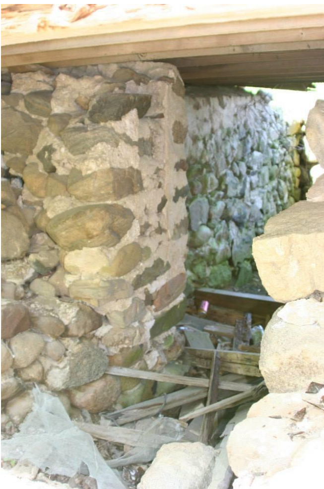
This is the southern side of the house and you can see how far it has been oved off the foundation. Again, kids were camping out in it at night in this state of maintenance
